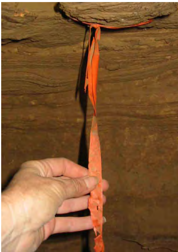
Figure 2: Deteriorating survey flagging tape.
