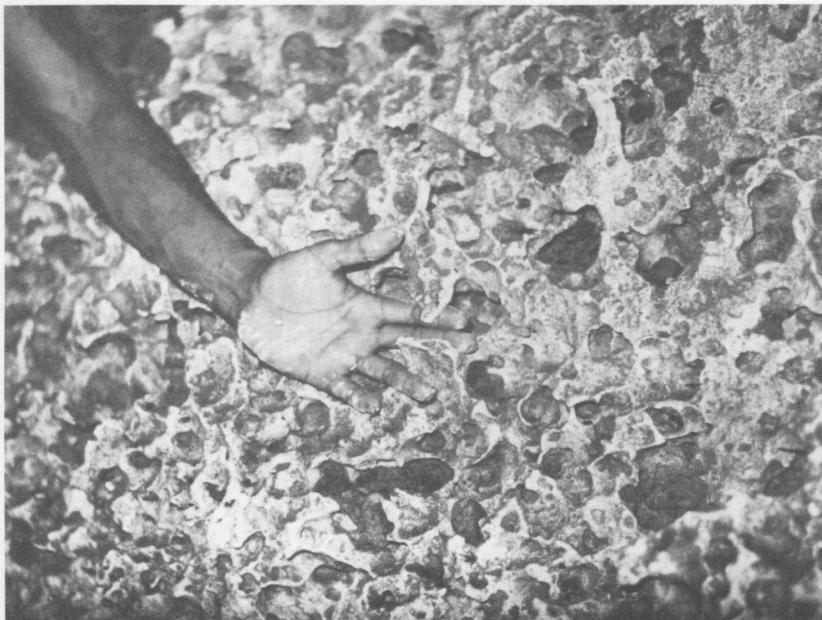
Plate 2. Carious weathering pits partially filled with clay, in the middle passage of Damawewe Cave.
