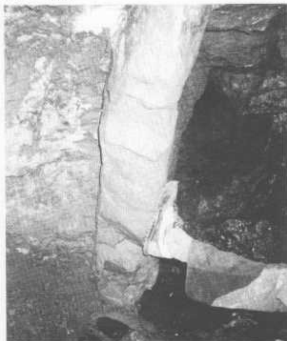
Figure 4. Outcrop of dyke in the Low Tunnel (most northerly dyke in Figure 3). Note how the side passage has developed along the upstream face of the dyke.
